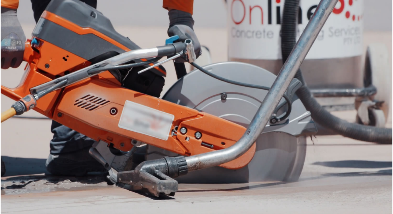
Image 4: Concrete cutting and clean-up using on-tool water suppression, dust extraction, and vacuuming.
